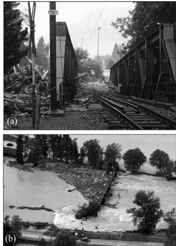
Figure 1. Drift accumulation at (a) railway bridge in Sarnen and (b) weir Perlen in Lucerne, during 2005 flood event in Switzerland, flow direction from left to right
