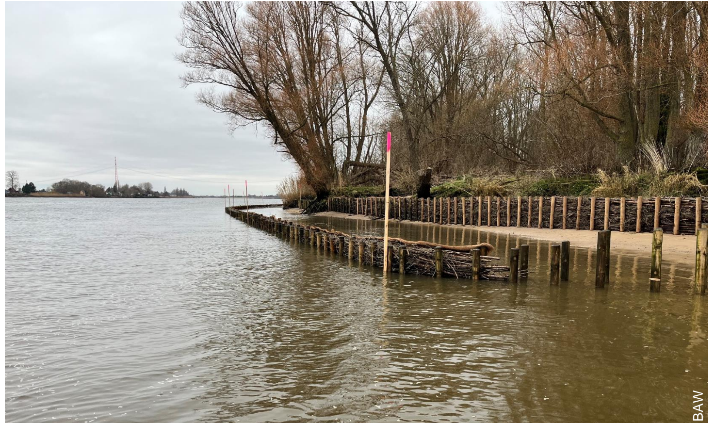
Construction of the brushwood boxes in December 2025. At the time the picture was taken, the area between the brushwood boxes had not yet been filled in and the edges of the boxes had not yet been completed.
