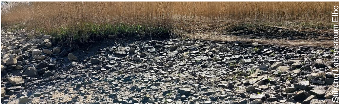
Measure at the beginning of 2023. Many of the underlying stones have been uncovered.
