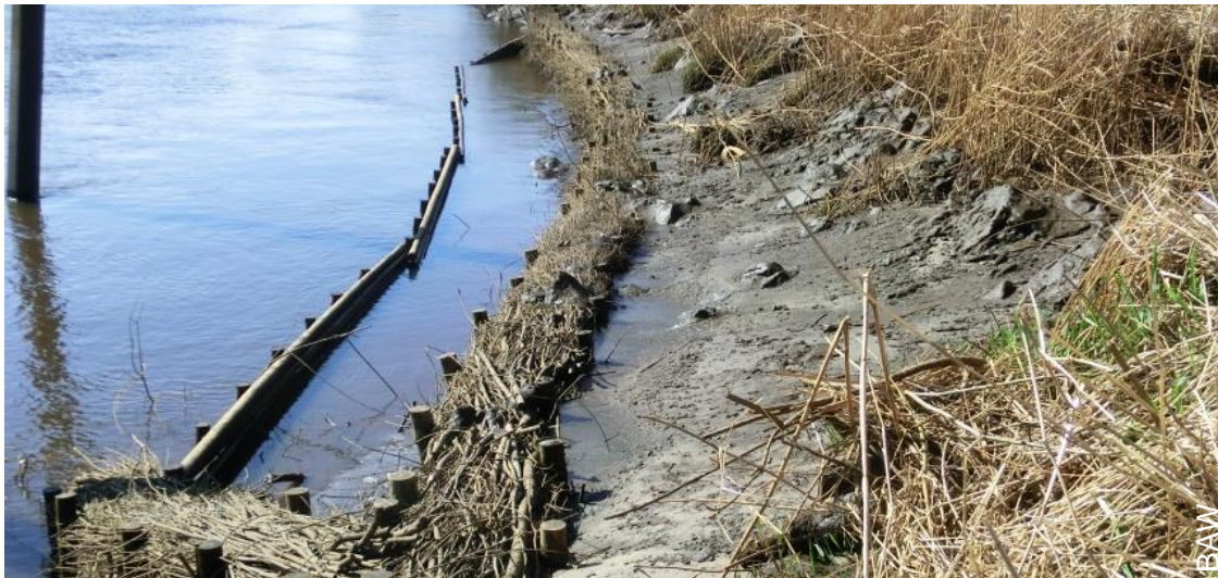
Pilot site 3 at the Wümme: Brushwood box with behind a pile wall in 2014.
