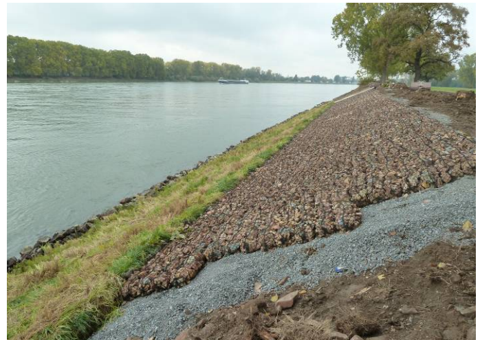
Figure 3: Test field with reed gabions (at the water-line) and stone mattresses on a granular filter layer on the upper slope
