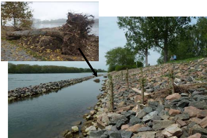
Figure 6: Stone wall with shallow-water zone and structural elements in the water and slope zones (dead wood trunks with roots, willow branch cuttings)
