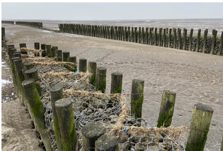
Figure 4: Condition of gabion boxes after ten years. Small damages to wooden piles. Source: BAW.
