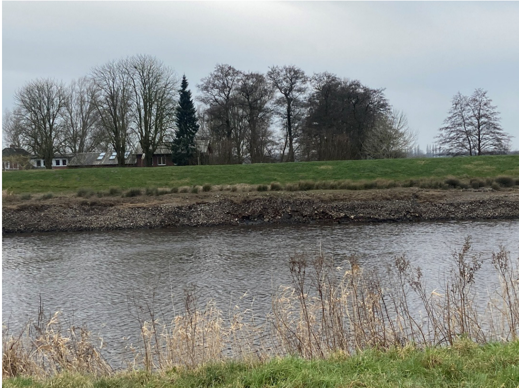
Figure 5: Damage to a rock armour revetment: Erosion of armour stones. Source: BAW.
