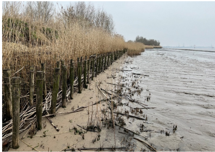
Figure 2: Typical damages of brushwood boxes: Degradation of filling. Source: BAW.
