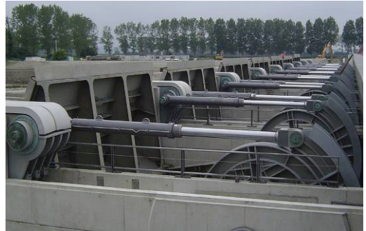
Picture 4 : all the hydraulic jacks seen from the abutment of the dam [J.Aubonnet]
