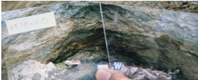
(erosion in the west side, April 3, 2009)
