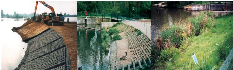
Figure 2. Articulated revetment mats, Hand placed concrete blocks, Established vegetation within the concrete blocks.
