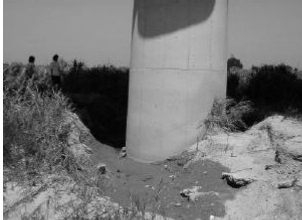
Figure 3. Local scouring around bridge pier in Ishige site (2002/8/8)
