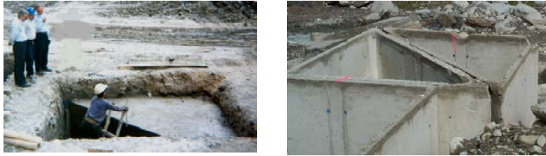
Figure 8: Prisms construction methods, without using sides' formwork and reinforcement (left), precast formwork filled with mass concrete (right)
