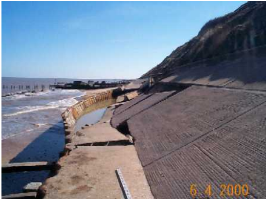
Figure 2. Seawall damage on the east coast of England (photograph courtesy of Waveney District Council)
