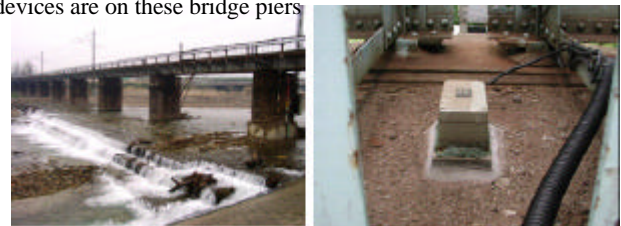
Fig.4 Clinometric type scour monitoring device.
