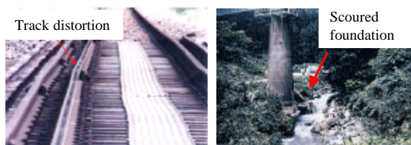
Fig.3 Site-situation of scour hazard occurred in 1995.
