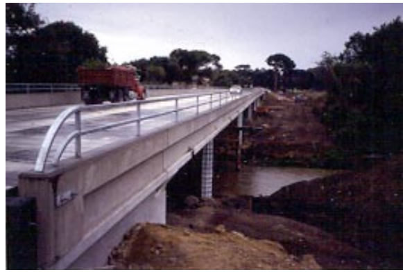
Figure 8: New Highway 1 Bridge with Pier Wall Construction under way (photo by Author, 1995)
